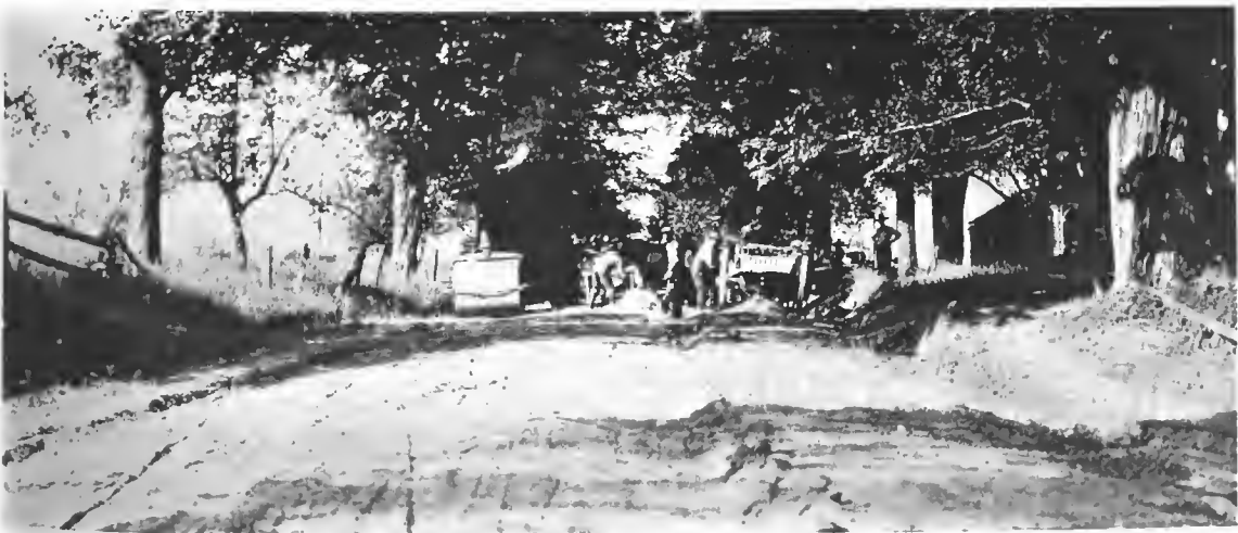
Some of the Actual Work of Road Building in New York State That Was Inspected by the Conventioneers.
